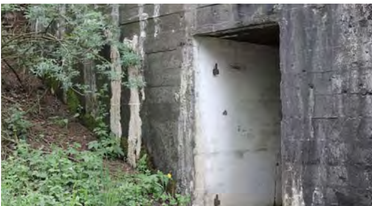
The road to the bunker and the entrance of the hospital bunker in the old refugee camp in Rom, Lemvig
